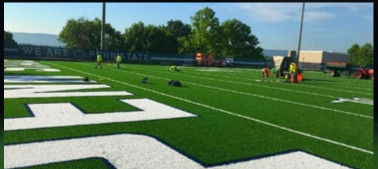
Stahl Sheaffer provided site engineering for the Lasch Field synthetic turf replacement in University Park, PA
